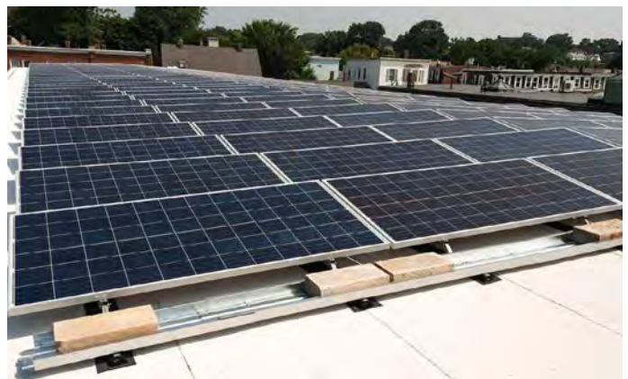
In net-zero energy buildings, renewable energy is generated on-site to provide for the building's total annual energy demand, such as through solar arrays.
